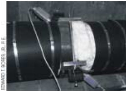
(c) Clamp-on hardware installed on a steam pipe; clamp due to Jim Hurd and John True; photo courtesy of Ted Borer.
