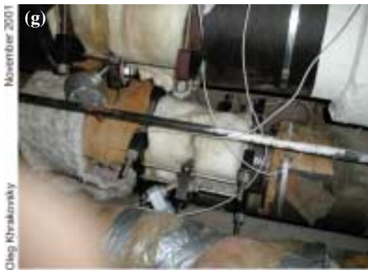
Clamp-on transducer installation on a 6" sch 40 carbon steel steam pipe @ 205 psi and 440°F inside steam distribution tunnel at Princeton University.
