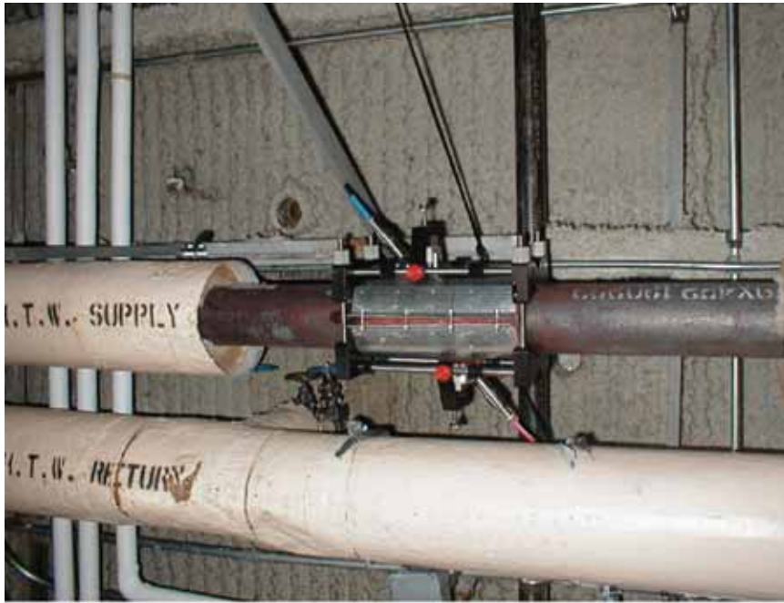
Clamp-on steam ultrasonic flowmeter installation on 4-inch CS Sch 40 steam supply line at the Living and Learning Building at the University of Vermont.
