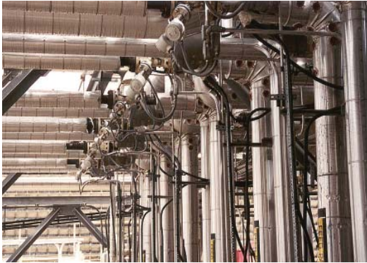
Flow meters installed on the vacuum distillation column feed
